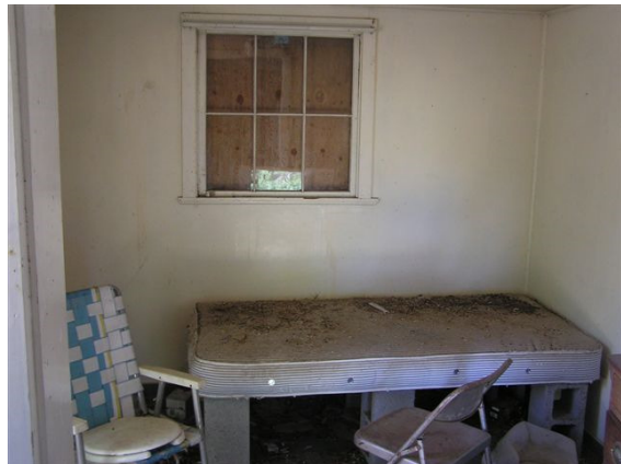
Figure 7. Condition of Sleeping Area
