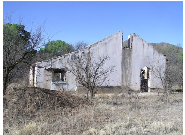
Wilbur Ranch House – Photo taken by T. Johnson after building was gutted and lost its roof.
